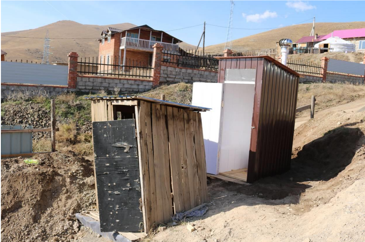
Construction of a new latrine for a family with a disabled child
